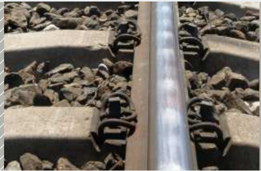
Rail corrugation (long wave)
